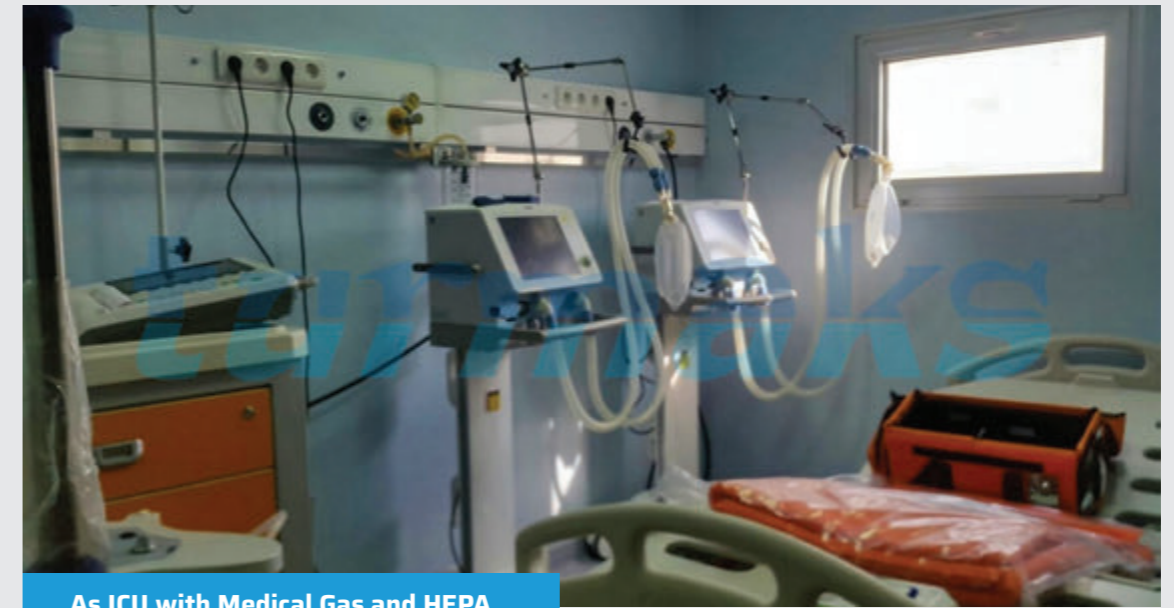
As ICU with Medical Gas and HEPA
