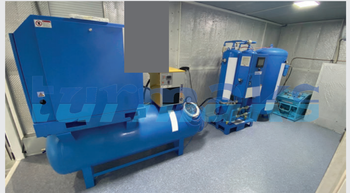
OXYGEN GENERATOR WITH CYLINDER FILLING SYSTEM
