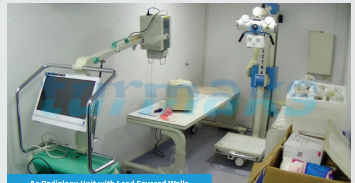
As Radiology Unit with Lead Covered Walls
