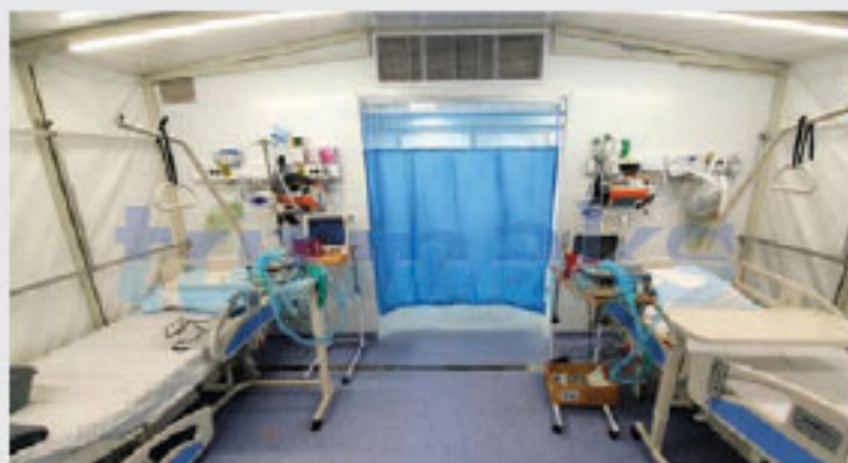
Integrated Medical Gas and HEPA filtered AC integrated
