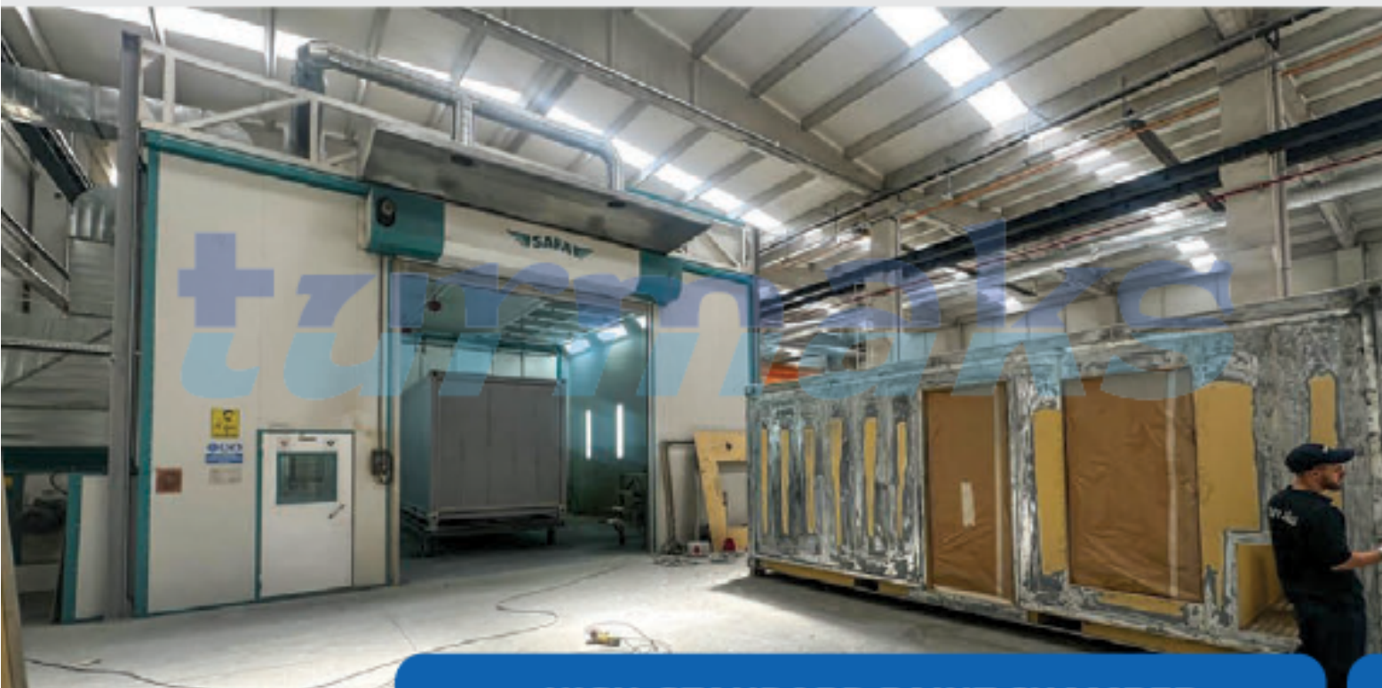
HIGH-STANDARD PAINT CHAMBER
