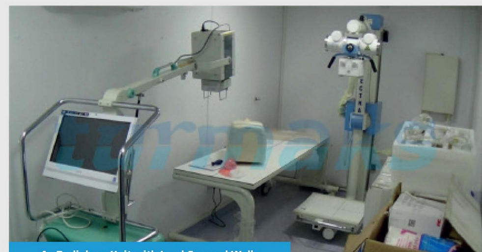
As Radiology Unit with Lead Covered Walls
