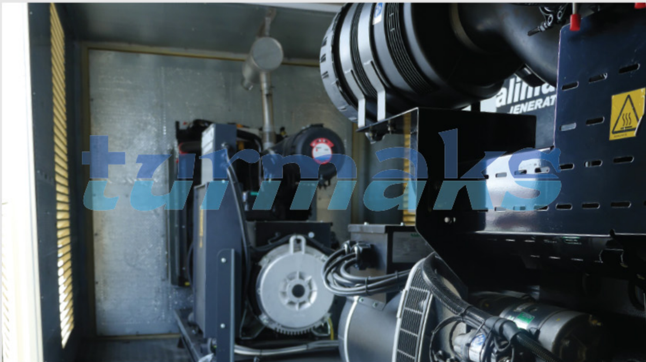
POWER GENERATOR SET WITH BACK-UP, CO-AGING AND SYNCHRONIZATION
