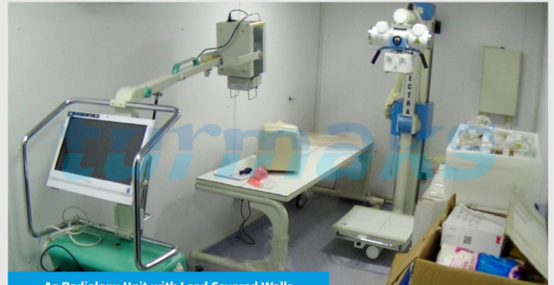
As Radiology Unit with Lead Covered Walls
