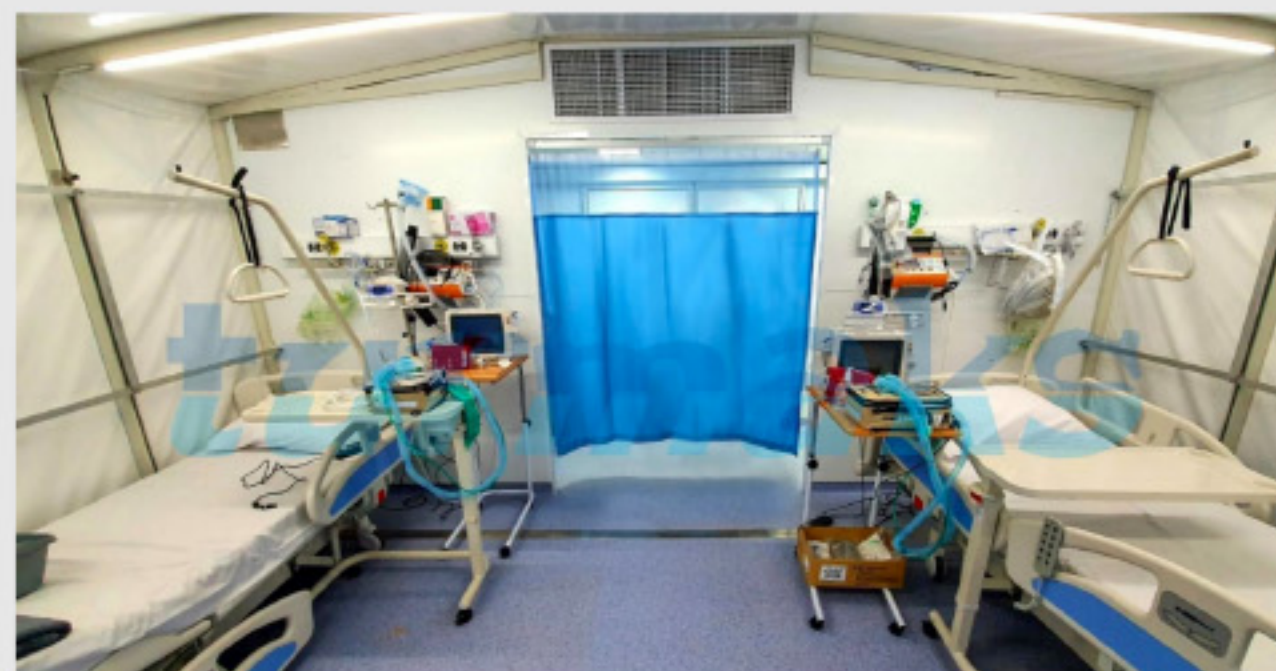
Integrated Medical Gas and HEPA filtered AC integrated
