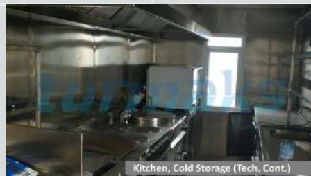
Kitchen, Cold Storage (Tech. Cont.)
